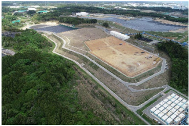
Soil storage facility at Interim Storage Facility (Okuma Town)
